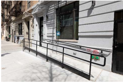
Handicap entrance ramp
