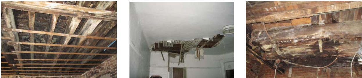
Images of existing wood joist and ceiling heavily deteriorated and damaged
